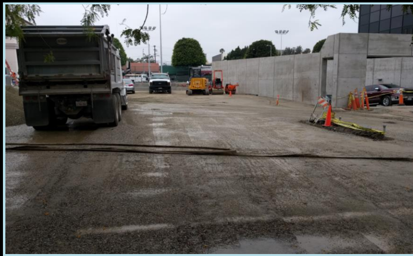
Base for Temp Portables
